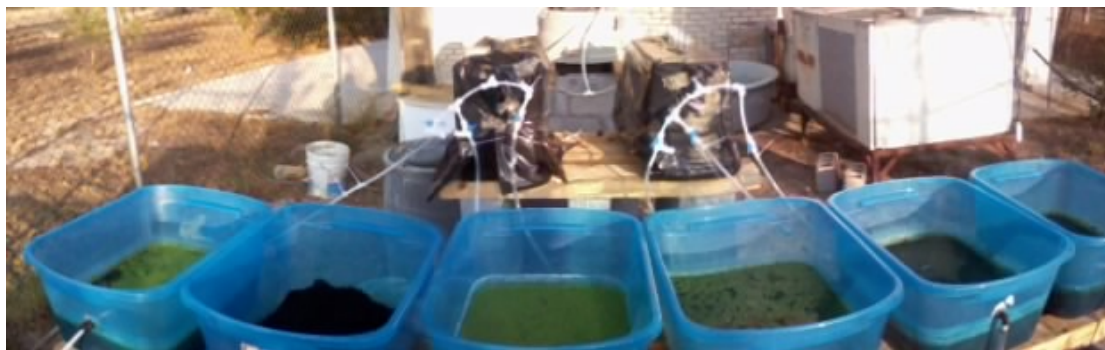
Figure 1. System hybrid for wastewater constructed in this project.
